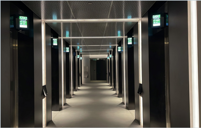
Photo of a lift lobby at a typical office floor during testing of "OEO" (courtesy of PMV).
